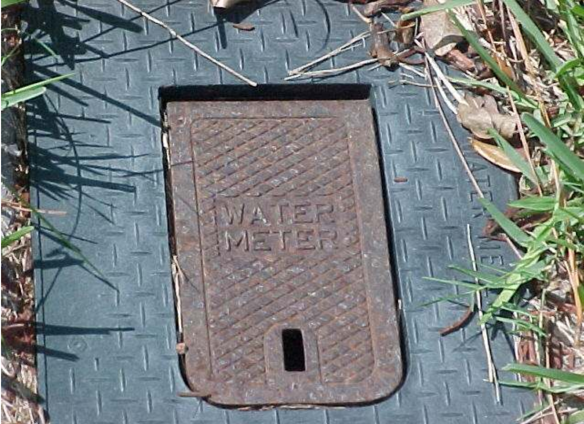
Typical water meter cover
